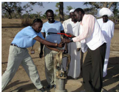
Workers repair a hand pump for water in South Sudan: infrastructure should be a top priority.
