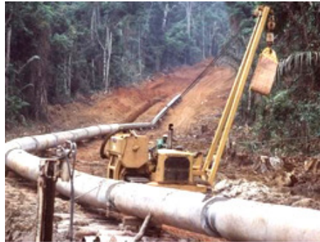
Construction of the oil pipeline: relying on the good intentions of the Chadian Government. Jans Kusters / Greenpeace
